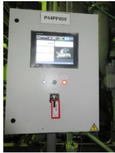
Figure 8. Redundant Local Control Unit
